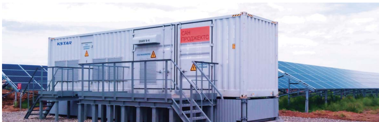
Russian 300MW PV Plant
