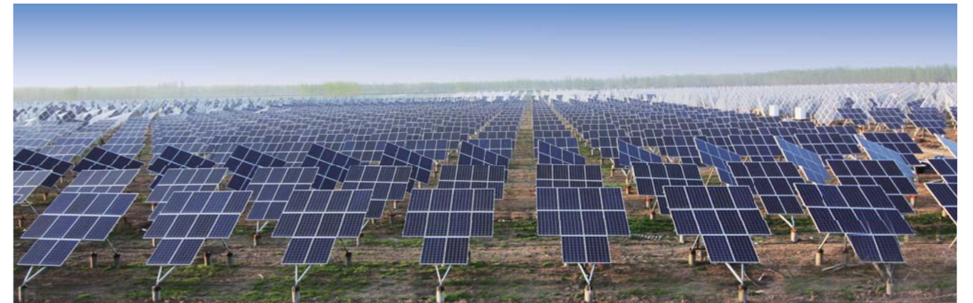
Jiangsu Tracking System PV Plant
