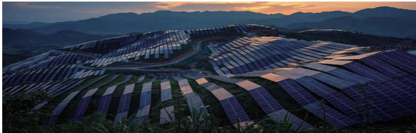
CGN Sichuang 50MW PV Plant
